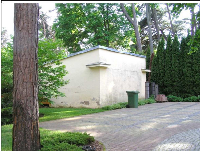
AS „Sadales tīkls” 10/0,42 kV transformators TP-160
